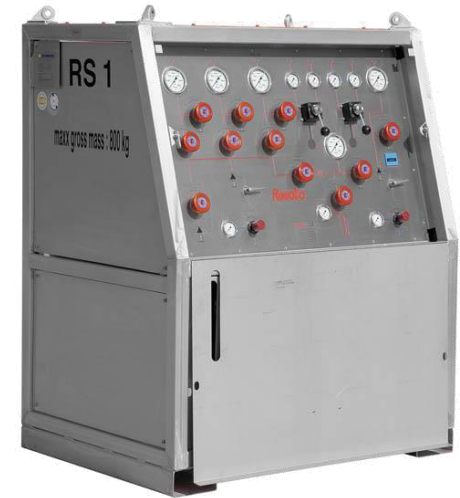
Multi line control panel
